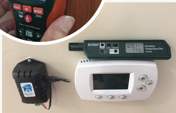
Above: Wood moisture content of bookcase measured at a moist 20.8. Below: Conditions inside apartment were 69% RH and 78°F.
