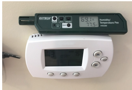
Conditions inside apartment were 69% RH and 78°F.
