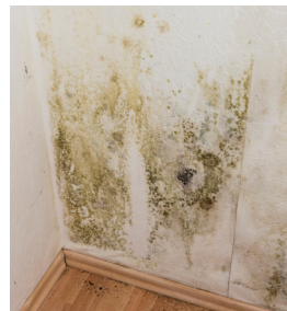
Mold growth on an interior wall.
